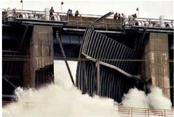
Folsom Dam Floodgate Failure, 1995
