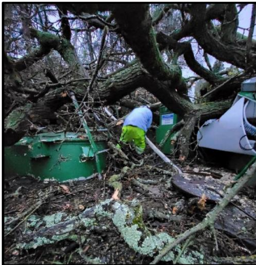
Figure O-6 Damage to S067 Pump Station, March 10, 2023
