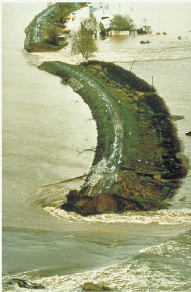
Figure R-19 1986 Tyler Island Levee Breach
