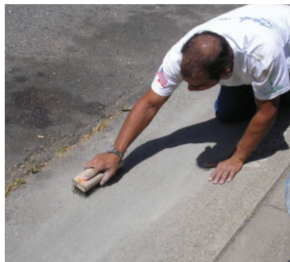
Illicit Discharges must be cleaned up immediately to keep pollutants from flowing into nearby storm drains and into creeks and rivers.
